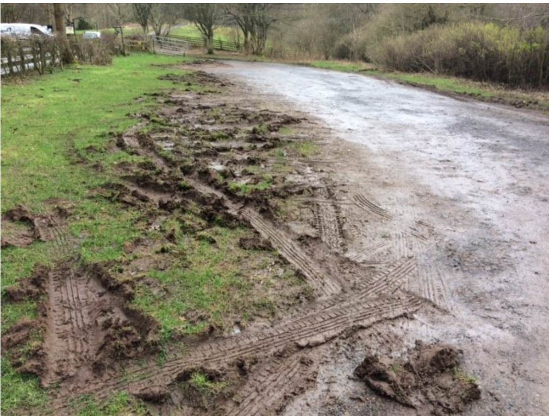
Figure 6 Overflow area acquired in 2019, unusable in wet conditions due to unbound surface
